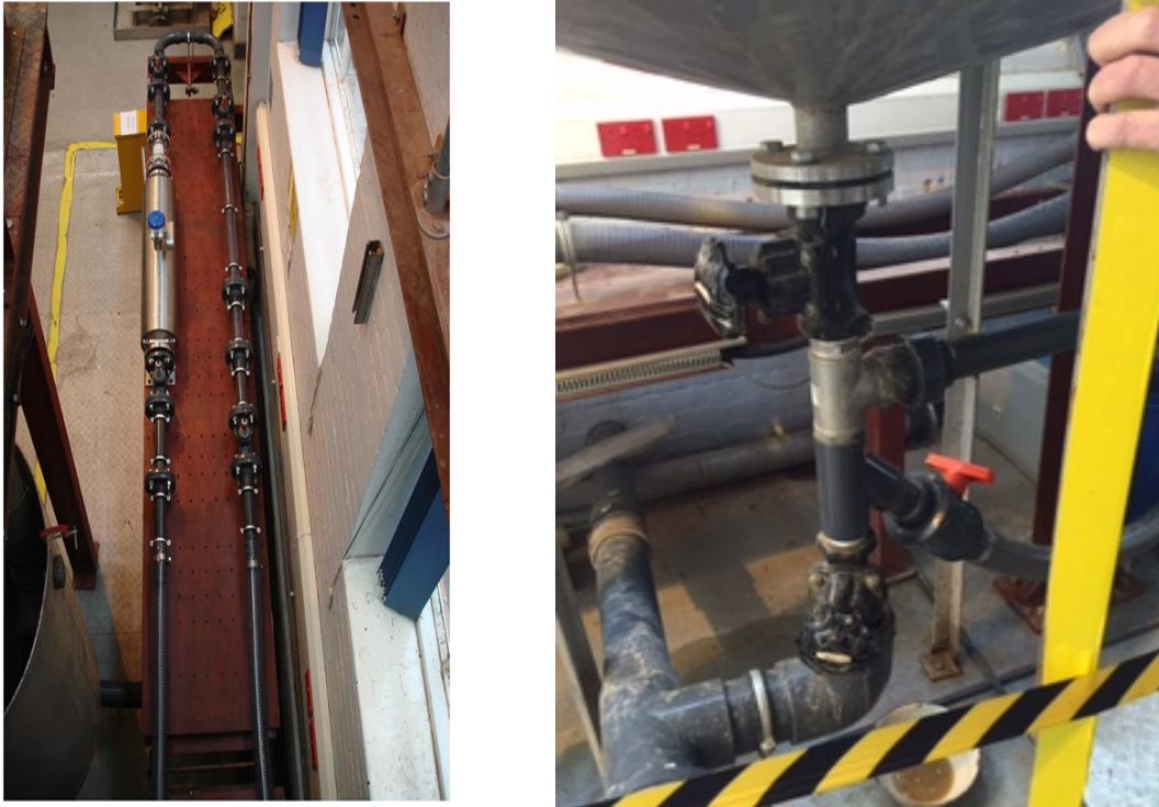
Figure 7: Coriolis mass flow meter (CMF), slurry mixing tank
